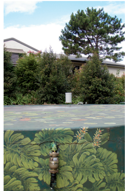
Water meter and rain gauge on communal tank, Capo di Monte
