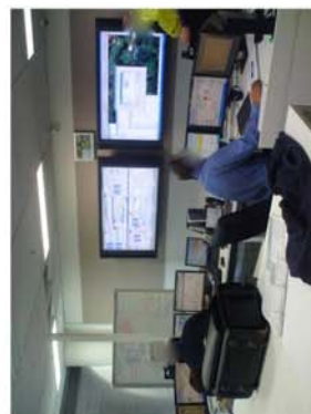
Figure 1. LinkWater Control Room
