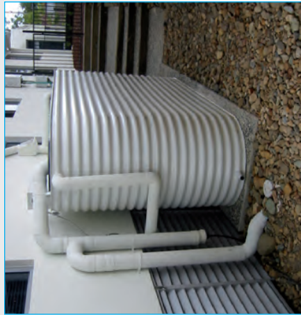
Beal, C., Gardner, T., Sharma, A., & Barton, R. (2010). A desktop analysis of potable water reductions from internally plumbed rainwater tanks in South East QLD. Urban Water Security Research Alliance Technical Report
