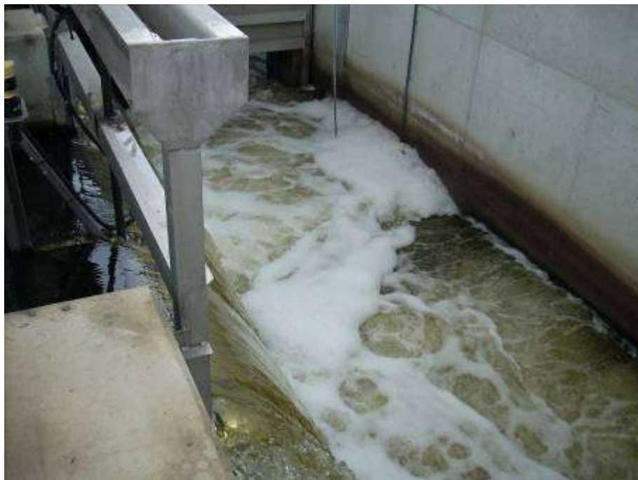
Figure 14 Oxley Creek WWTP post UV.
