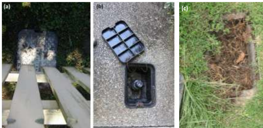
Figure 3: Examples of unsuitable water meter boxes.
