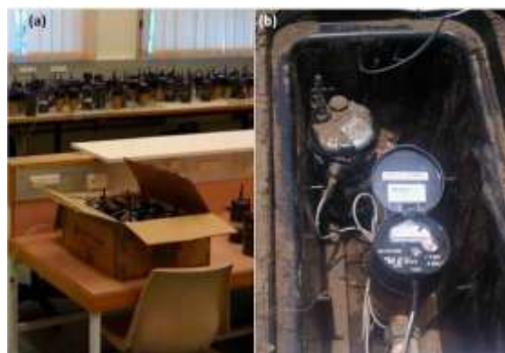
(a) Each meter/data set was individually configured. (b) Installed smart meter and data logger.
