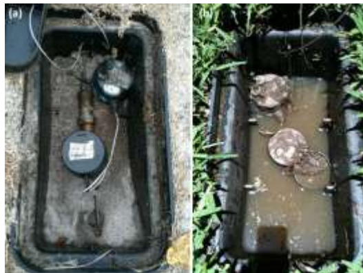
(a) Sand build-up in meter box. (b) Flooded meter box.
