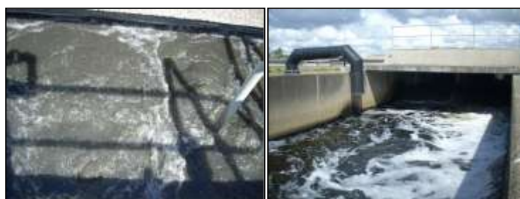
Figure 1. Sampling sites at Luggage Point Wastewater Treatment Plant.
