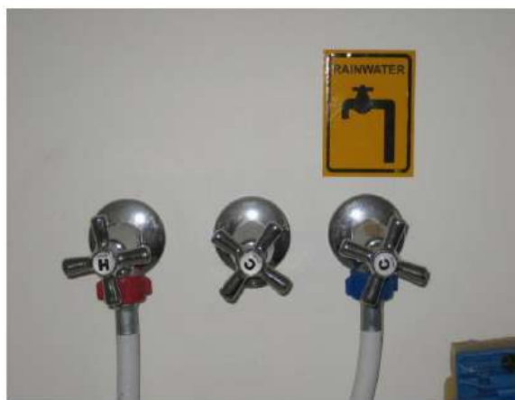
Figure 7: An example of the water supply connection to a washing machine. Note the dedicated rainwater tap as well as mains supplied hot & cold water taps.
