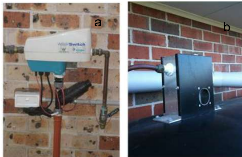
Figure 9: Mains back up water switching devices. The electronic switching valve device is shown in the LHS photo, whilst the mechanical trickle top-up device is shown in the RHS photo. The mechanical device uses a float and rod installed in the tank and connected to a mechanical valve located on the top of the tank.
