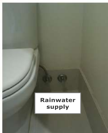
Figure 6: An example of a rainwater supply connection that fills the toilet cistern.
