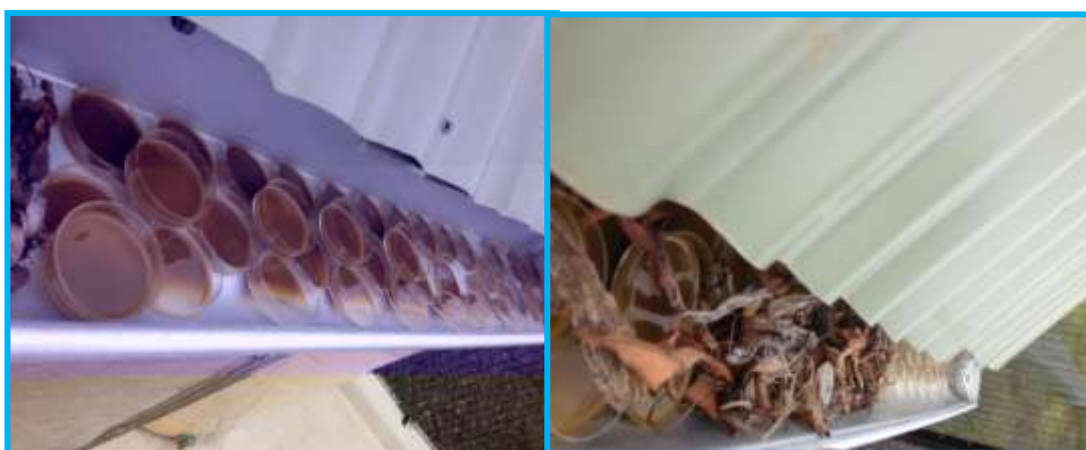
Figure 8. Possum faecal slurry in the gutter.
