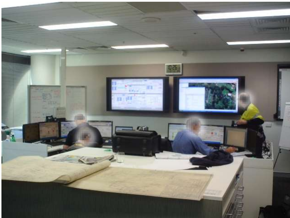
Figure 1: The control room at the BWTA central office, showing two operator consoles with four monitors each, and two large wall-mounted LED screens.
