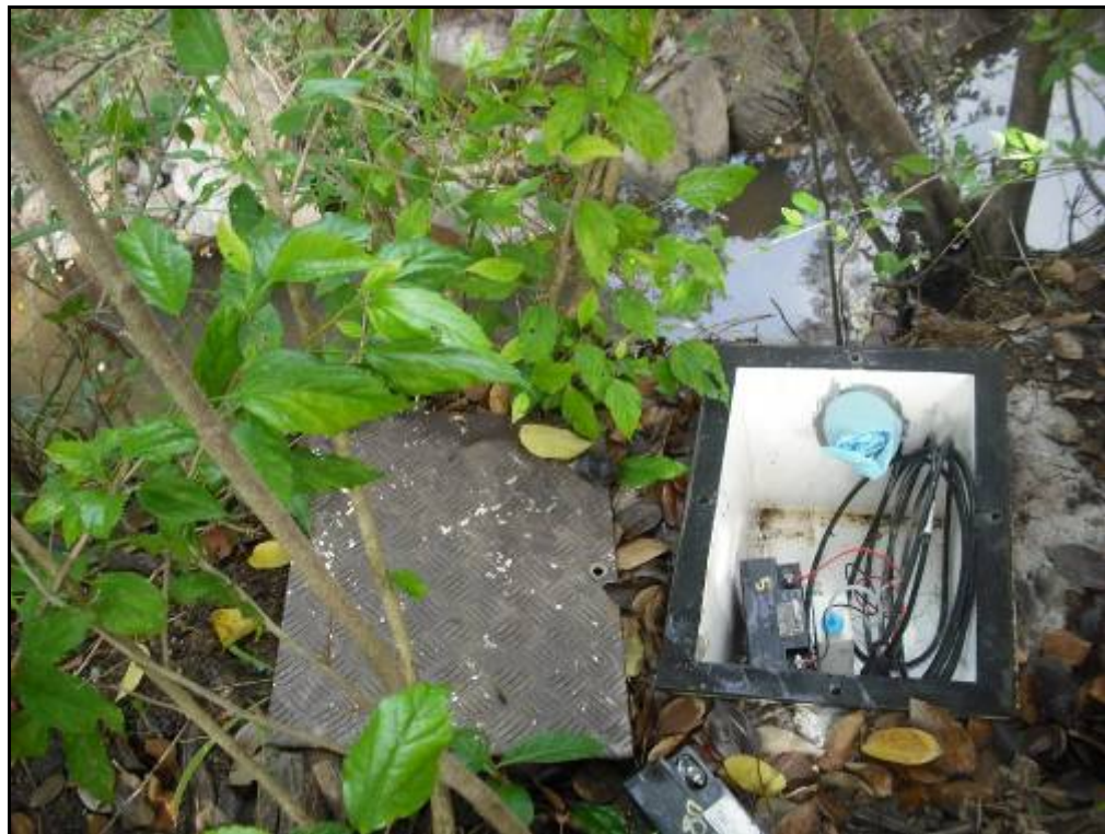
Figure 16: Replacement of battery of data logger / pressure transducer at Stable Swamp Creek, Sunnybank. The lid of the environmental enclosure is on the left of photo.
