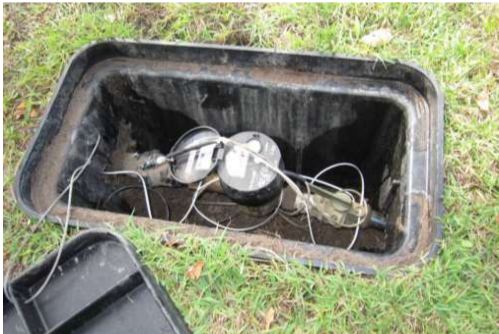
Figure 6: External utility water meter with cable connecting to CSIRO sensor module.
